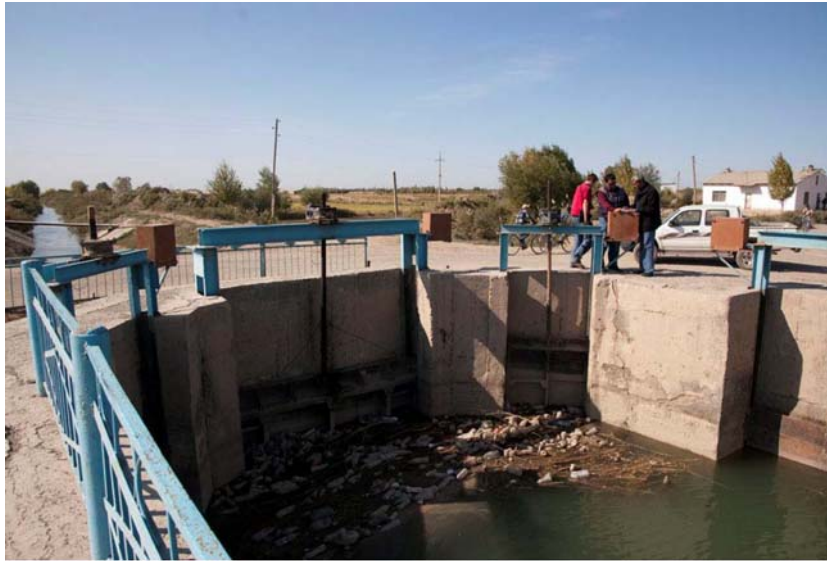
Control gates for regulating water distribution on a main canal system in Khorezm (photo courtesy of Dr. A.M. Manschadi)
